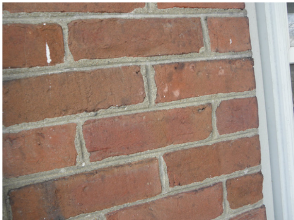
The masonry requires repair, a complicated process. Photo by Karen Schaefer.
