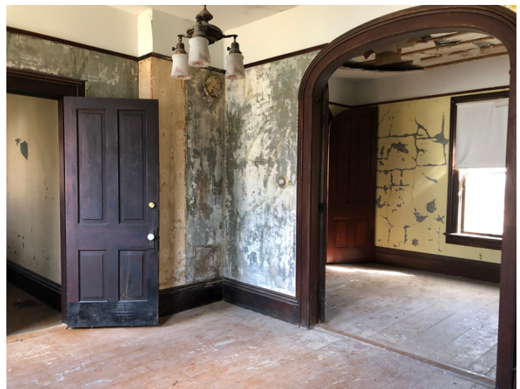
View of dining room with door to the front hall on the left and archway to back parlor on the right. Photo by Carol Lasser.
