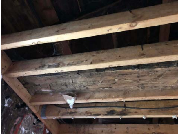
Ax-hewn beam discovered in ceiling of the kitchen wing. Photo by Carol Lasser.
