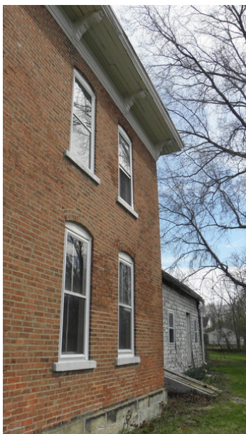
View of the east side of the Evans house showing the wooden "kitchen wing" behind the brick structure facing the street. Photo by Karen Schaefer.
