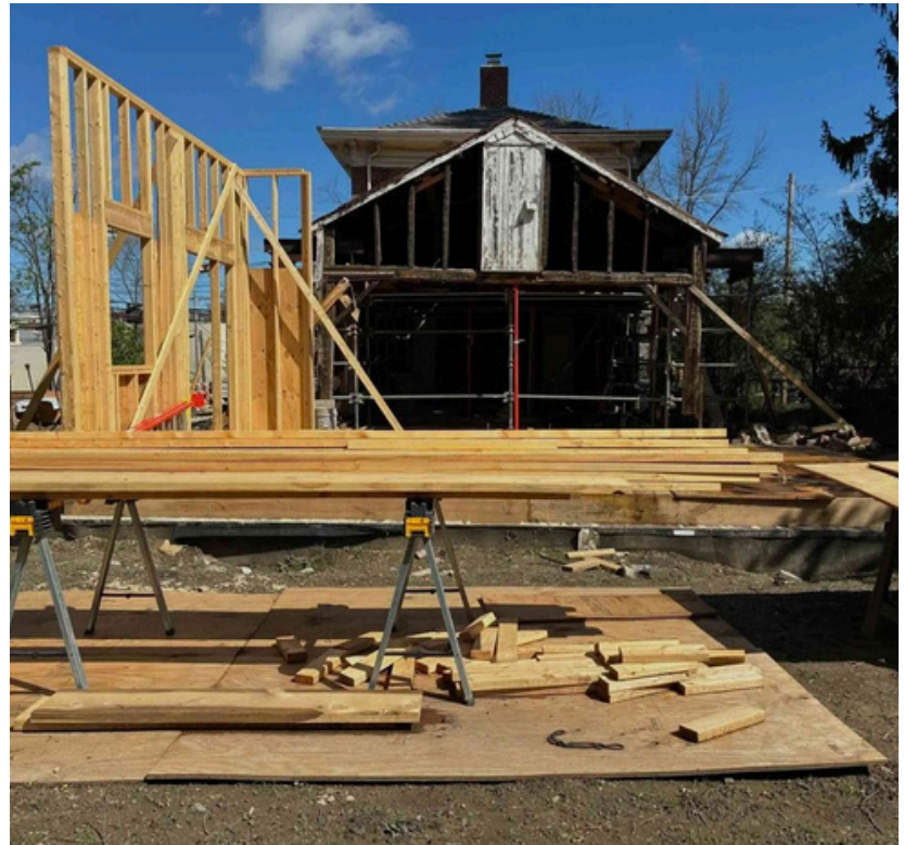
Rear view of the Evans House showing the original portion of the building undergoing rehabilitation and an emerging frame for the new annex. Photo courtesy of Carol Lasser
